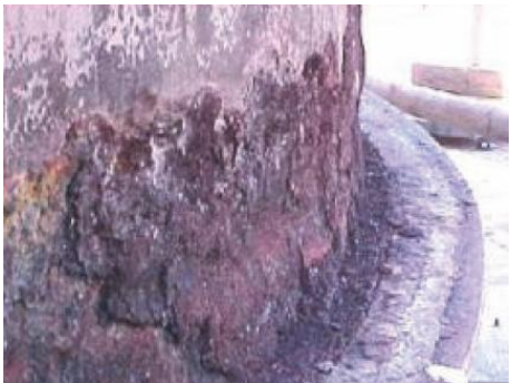
CUI at insulation support ring
