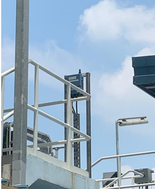
GATEWAY AT CONTROL ROOM ROOF
