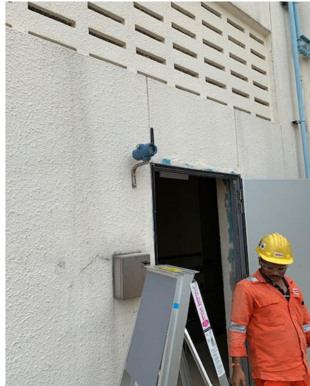
REPEATER OUTSIDE BUILDING
