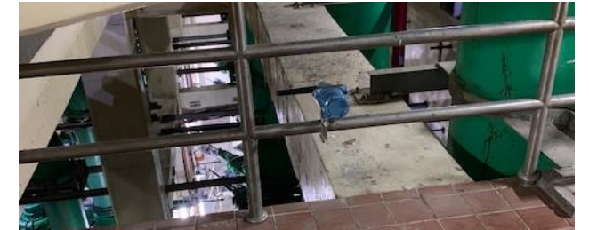
REPEATER AT BASEMENTS
