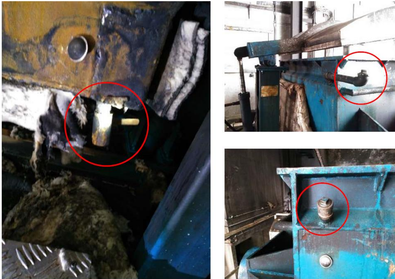
Figure 40: All three openings on the oil jacket circled in red were found closed
