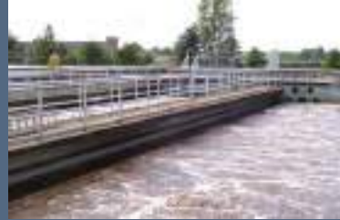
Biological process in Water Reclamation Plants
