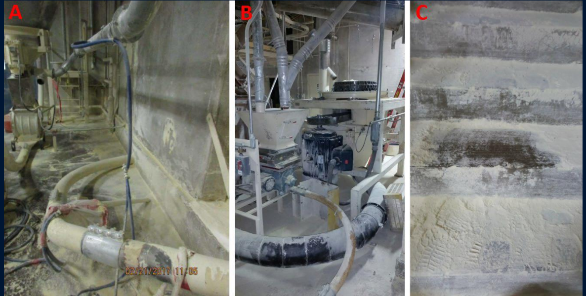
Examples of fugitive dust accumulations, (A) approximately three months before the incident, (B) approximately two weeks before the incident, and (C) less than 24 hours before the incident.
