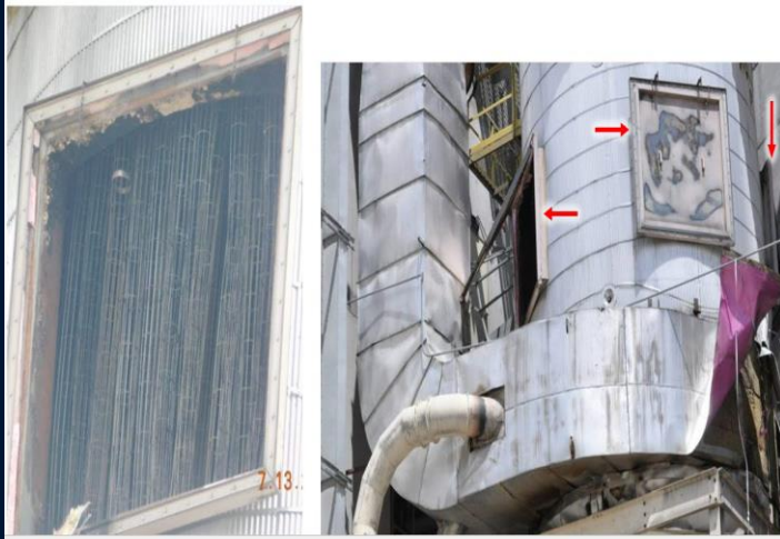
Dry Grit Filter damage. Internal damage (left). The filter socks were burned away, leaving only the metal cages. Deflagration vents (right, red arrows) stuck open and with burn damage. (Credit: Didion, annotations by CSB)
