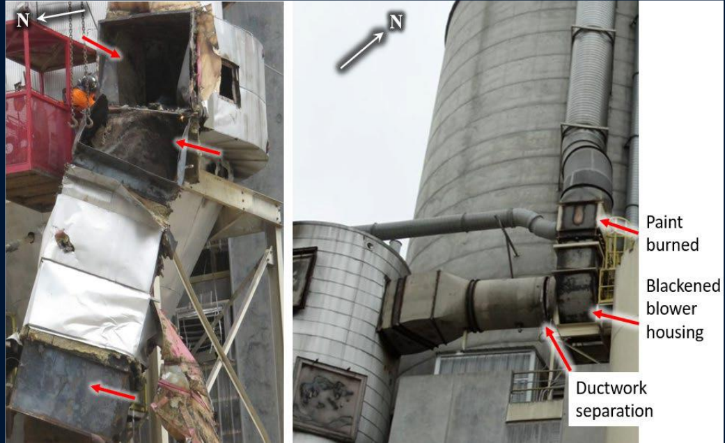
Examples of Dry Grit Filter ductwork and blower damage (red arrows). Inlet duct blackened (shown during demolition, left) and exhaust to atmosphere, including blower (right). (Credit: left, Didion with annotations by CSB; right, CSB)
