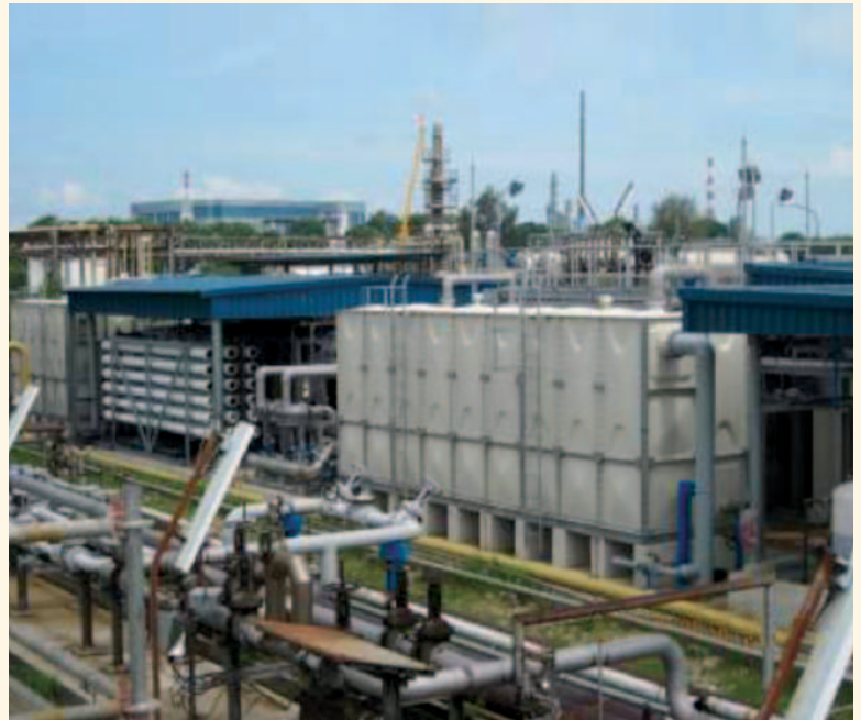
Figure 1: Effluent Water Treatment Recovery Plant (ETRP)
