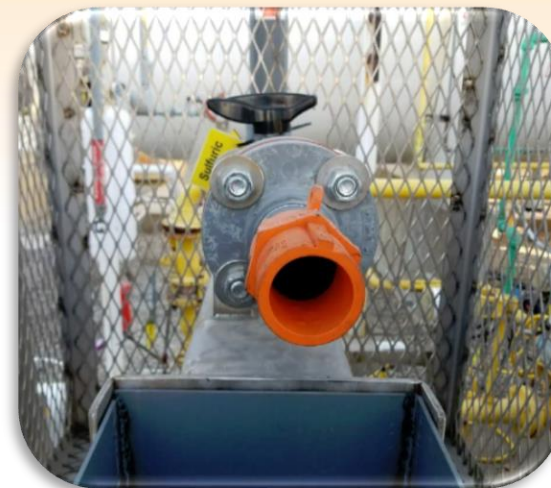
New coupling on the sulfuric acid fill line
