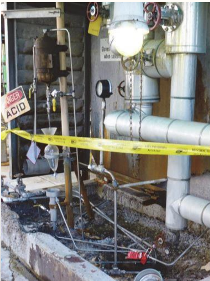
The sulfuric acid sampling station after the Feb 2014 incident.
