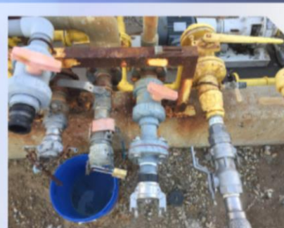
BEFORE: Old unloading portals (photo courtesy of CSB)
