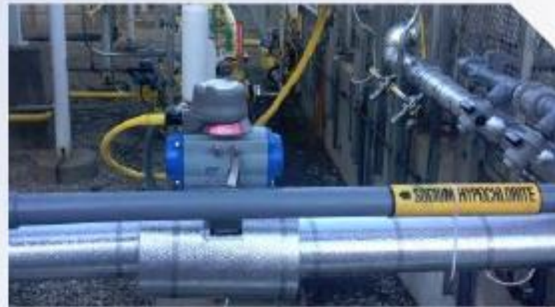
New shutoff valve (photo courtesy of MGPI)
