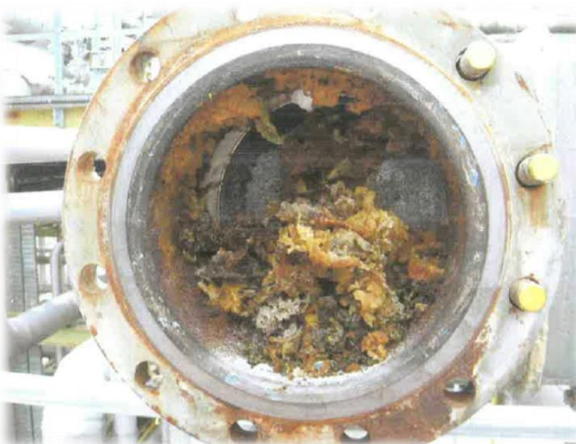
Pressure Relief Valve's Outlet Isolation Valve plugged with polymers
