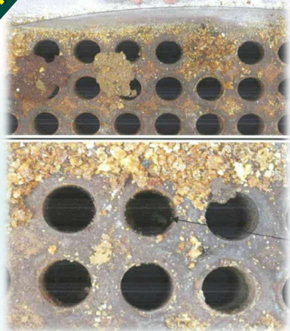
Reboiler Upper Tubesheet and tube inner wall – Brownish Rubbery polymers
