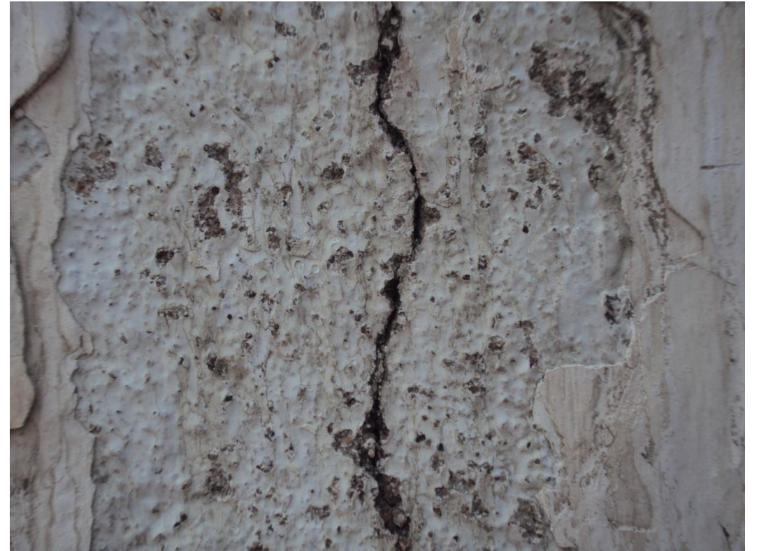
Crack in wall
