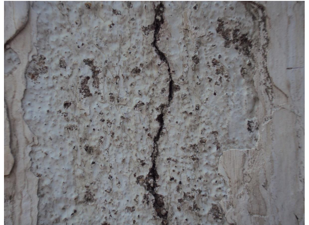
Crack in wall
