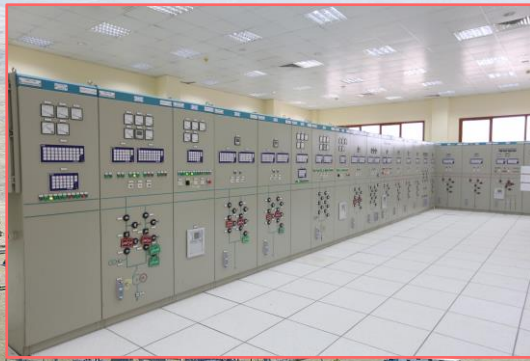
ELECTRICAL SYSTEMS AND SOLUTIONS
