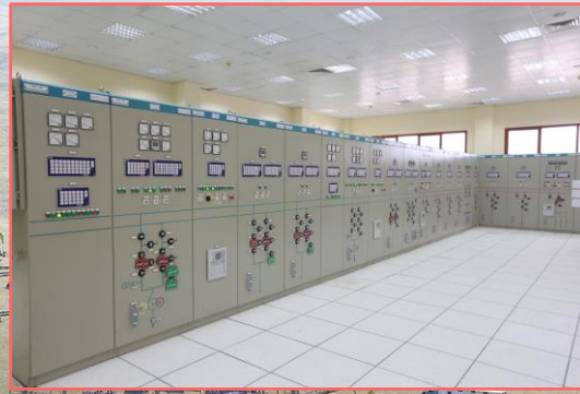
ELECTRICAL SYSTEMS AND SOLUTIONS
