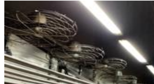
Ventilation at work area
